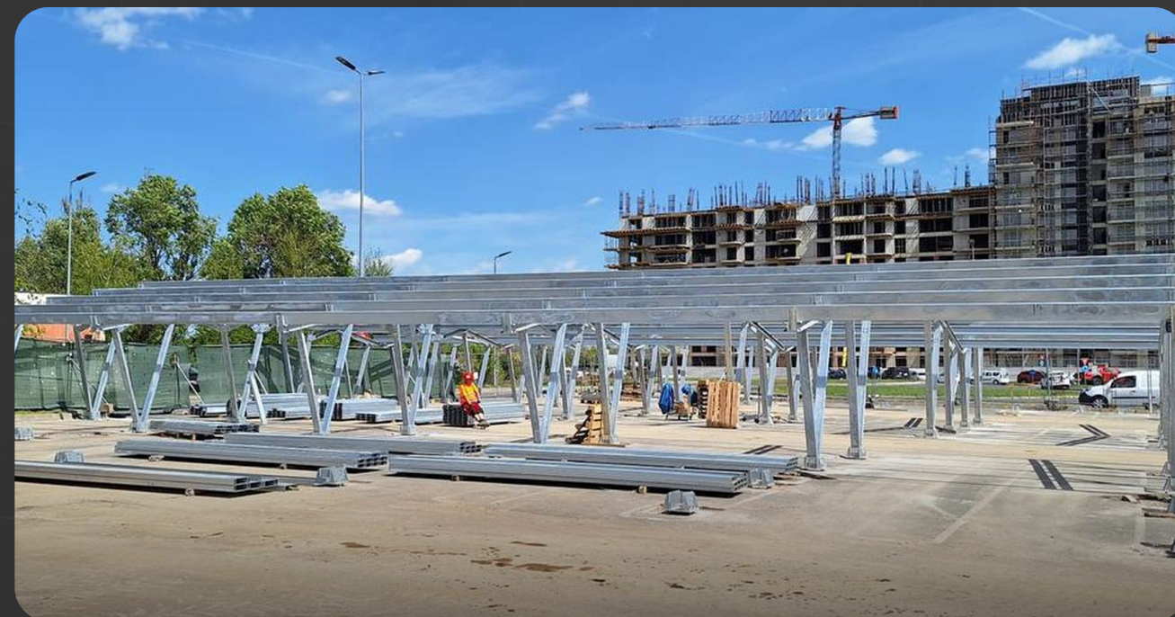
SOLAR CARPORT, MODEL W, 742.5 kWp
